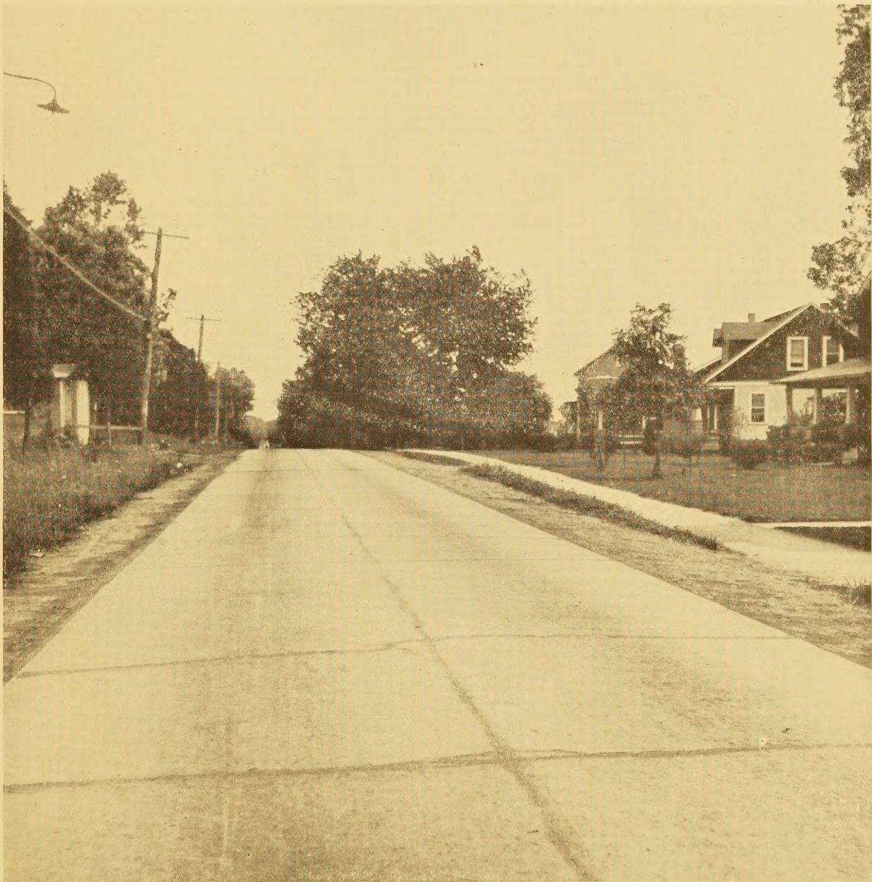
EXPERIMENTAL SECTION OF THE COLUMBIA PIKE SHOWING TYPICAL CRACKS IN A REINFORCED CONCRETE SURFACE
